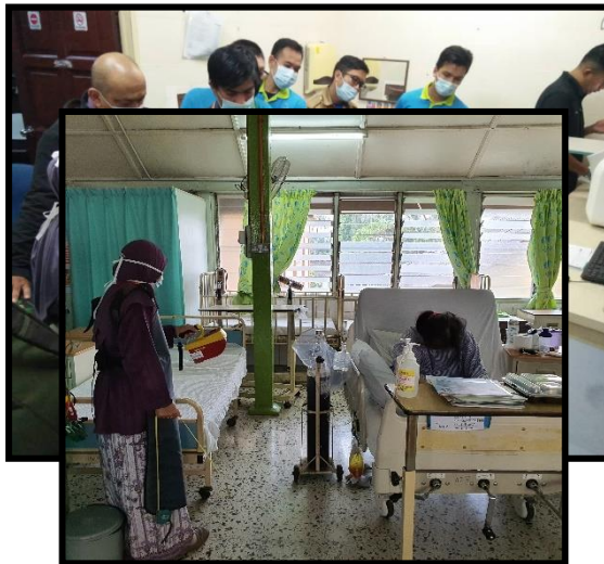
Testing & Commissioning (T&C) Computed Radiography (CR) System di Unit Radiologi Klinik
